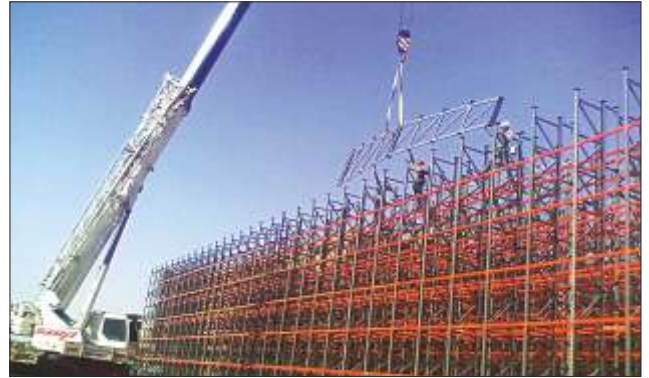
RSW, EGYPT (Under Installation)
